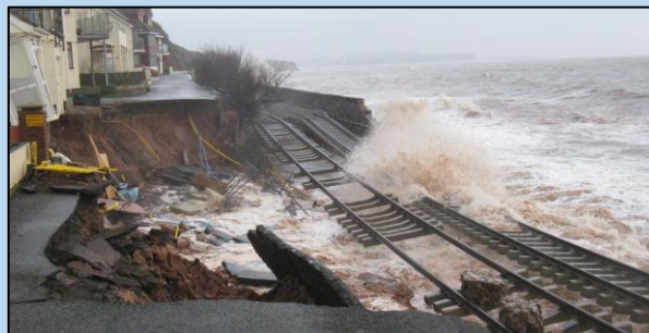
Damaged railway lines at Dawlish, 2014
