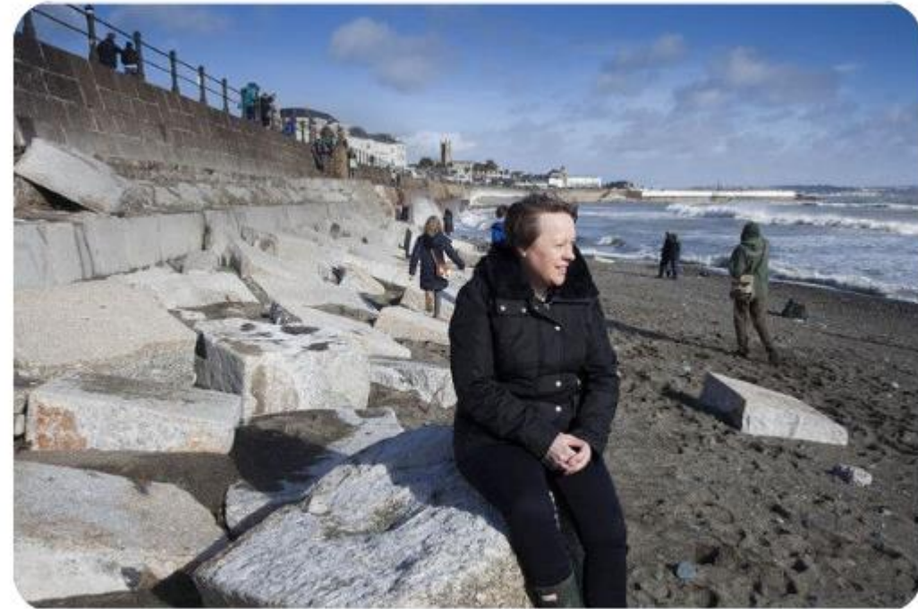
Penzance sea wall damage from Storm Callum – source Shadow environment secretary Maria Eagle surveys the storm damage in Penzance | Penzance, Bristol, Storm (pinterest.co.uk)
