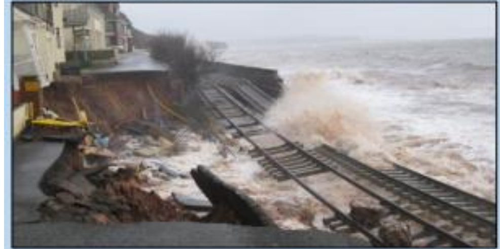
Damaged railway lines at Dawlish, 2014
