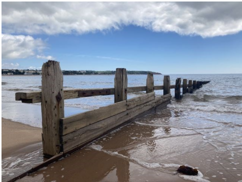
Old groyne at Dawlish Warren — photo: Paul Berry
