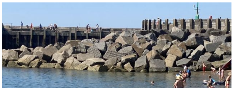
Rock armour, West Bay — photo: Paul Berry
