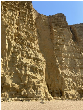
Joint collapse, East Cliff — photo: Paul Berry
