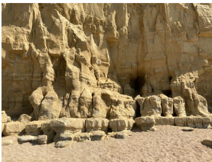
Marine erosion at the base of East Cliff — photo: Paul Berry
