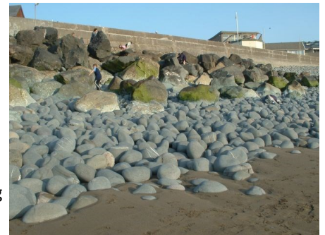
Storm beach pebbles in front of sea wall and sea armour —photo: Paul Berry
