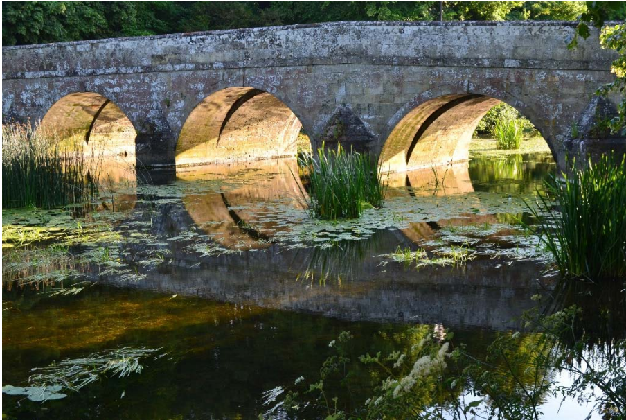
Blandford Bridge – built, widened and repaired in C18th and C19th, but there had been a bridge since C13th and a ford since Anglo-Saxon times.
